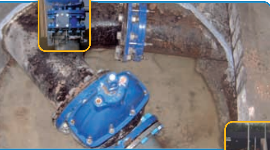
Right: entrance to the Conwy tunnel Above: the pipeline and valves, post remediation
